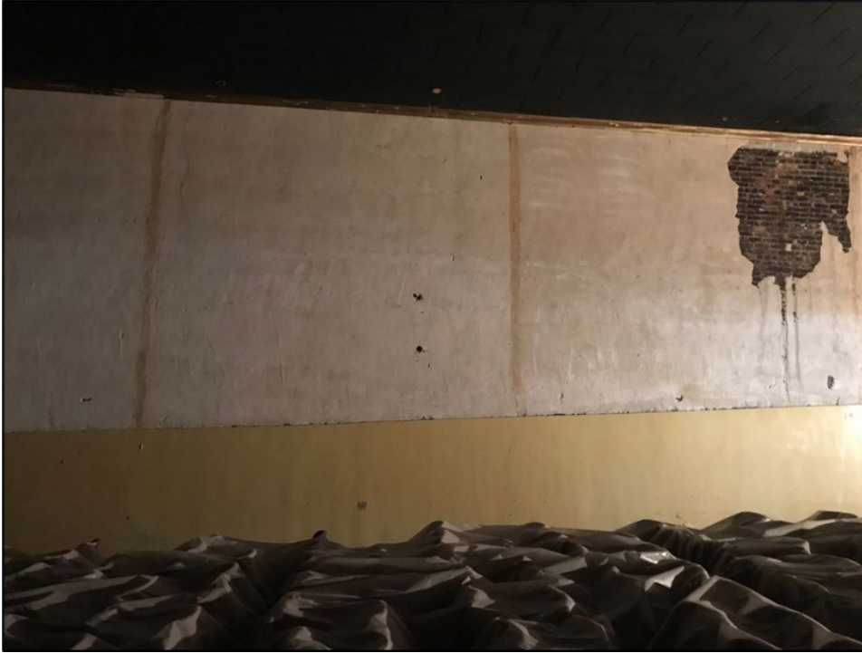
Photo 27 Charred wall in auditorium from electrical fire, facing south (2020)
